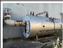
#58: Thermal Power Plant and Burner
