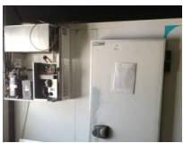
#3: Rivacold Cold Room
