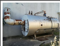
#58: Thermal Power Plant and Burner
