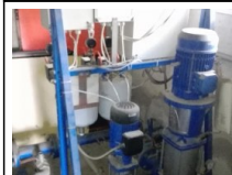
#47: Skid Bombas Contra Incendios Lowara
